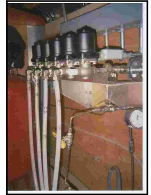
The system includes automated solenoid valves that allow pulses of ozone gas to be injected into six sparge wells.
