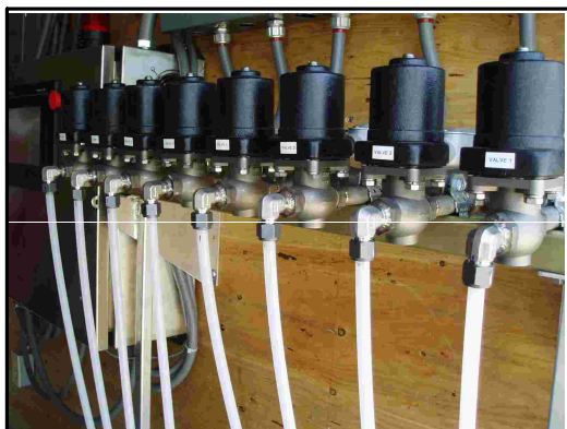
The system includes automated solenoid valves that allow pulses of concentrated ozone gas to be injected into eight sparge wells.
